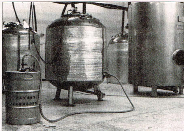
Six round-bottomed Grundy tanks serve as fermenters. They have cooling jackets welded to the outside.
