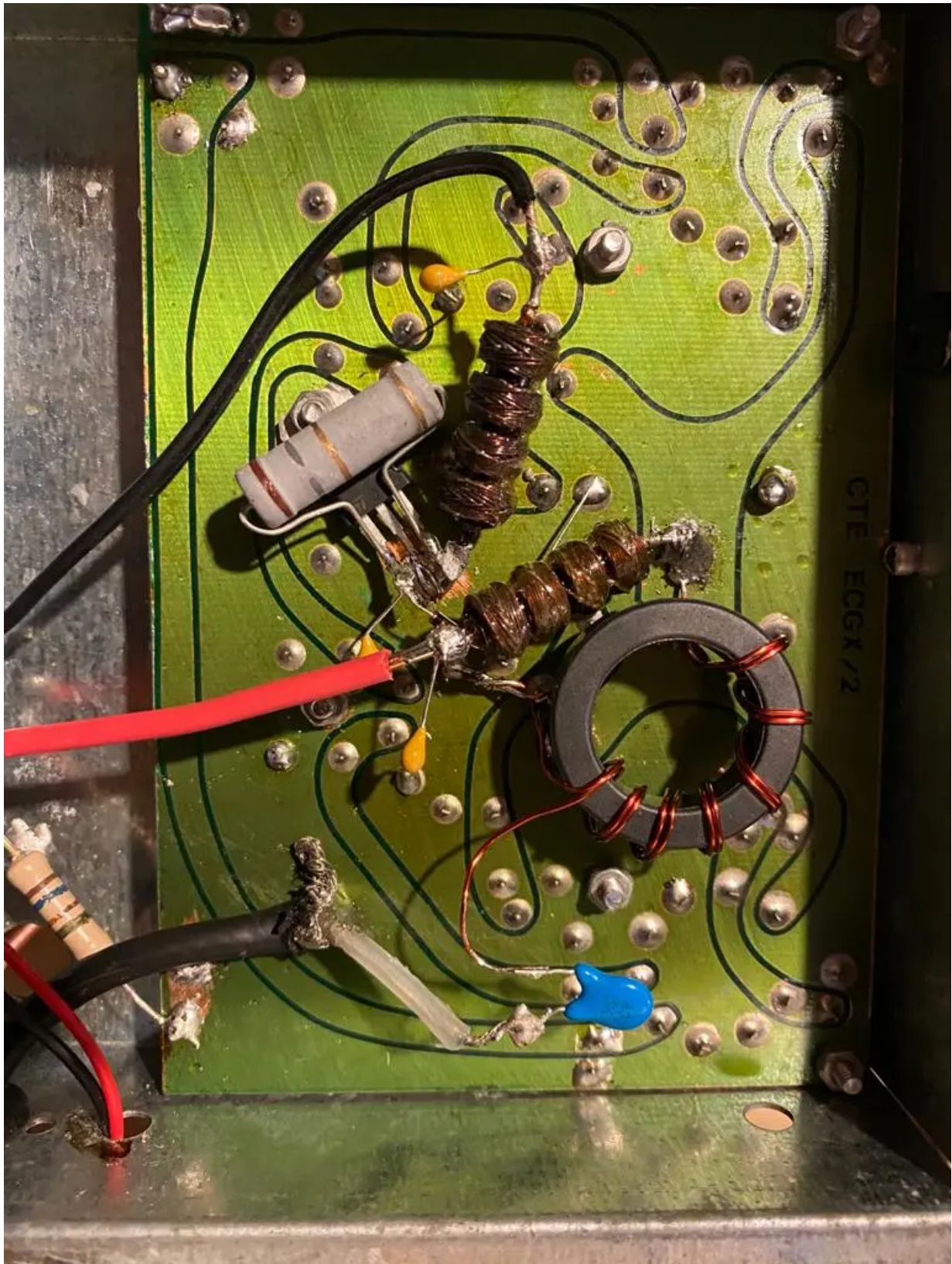
Biassing with the input transformer. The relay is not the picture and the 16k resistor is on the left of the picture. The BD912 is underneath the resistor
