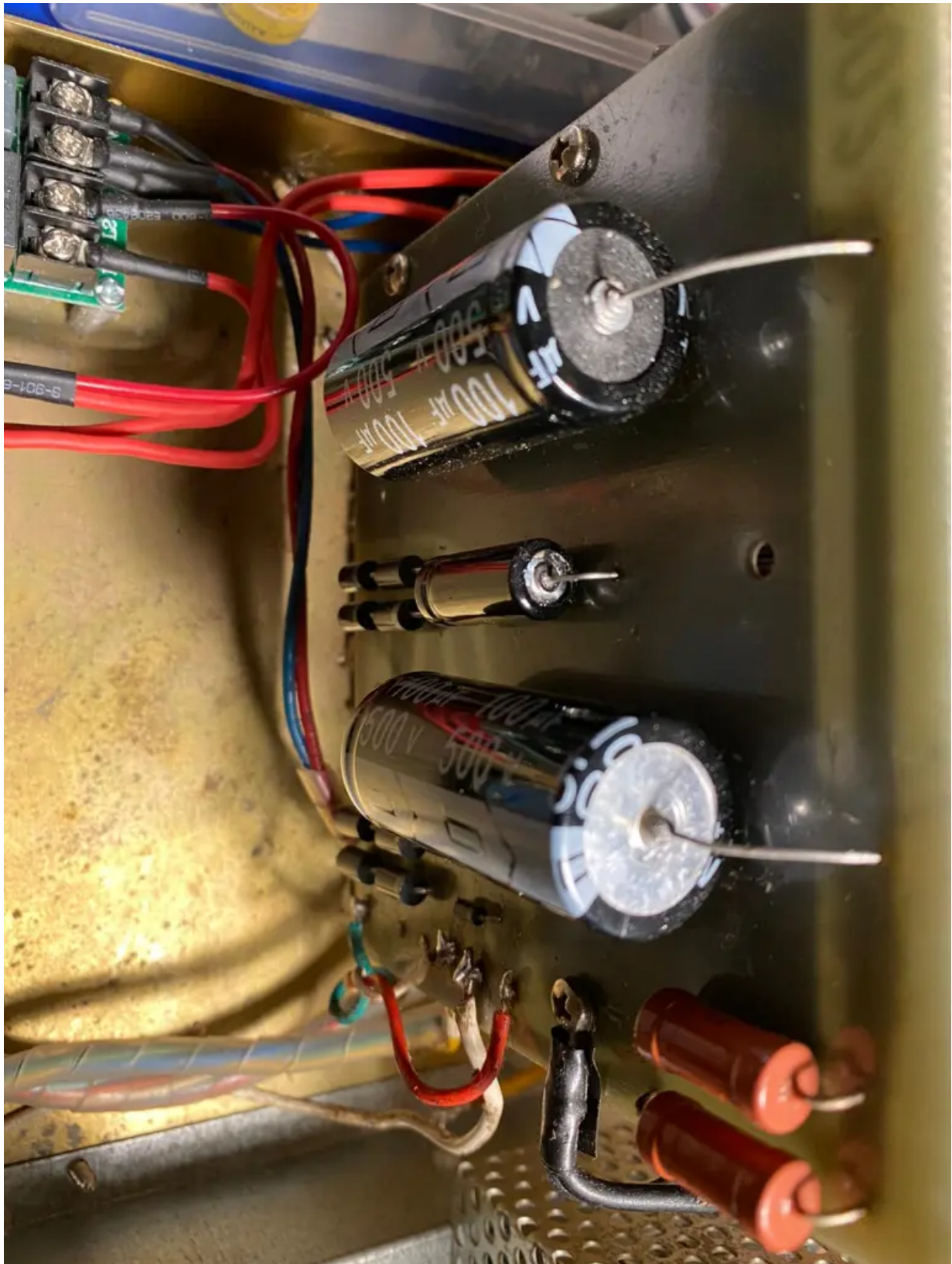
The high voltage PCB was totally refurbished with new Diodes and capacitor
