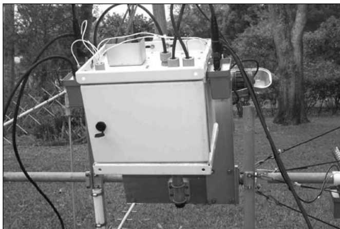
Figure 17.56 — A NEMA 4 box is used to shelter the L-band electronics and power supply. The box flanges are convenient for mounting preamplifiers. The box is shown inverted since it is on a tilt-over tower. (KD1K photo)
