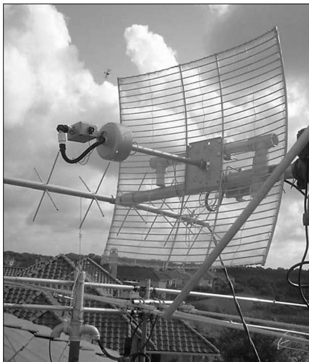
Figure 17.46 — Mesh modification of an MMDS dish antenna by K5OE, with a helix-CP feed and preamplifier by Down-East Microwave mounted directly to the helix feed point. (K5OE photo)
