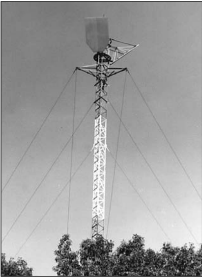
Figure 15.100 — Commercial periscope antennas, such as this one, are often used for point-to-point communication.
