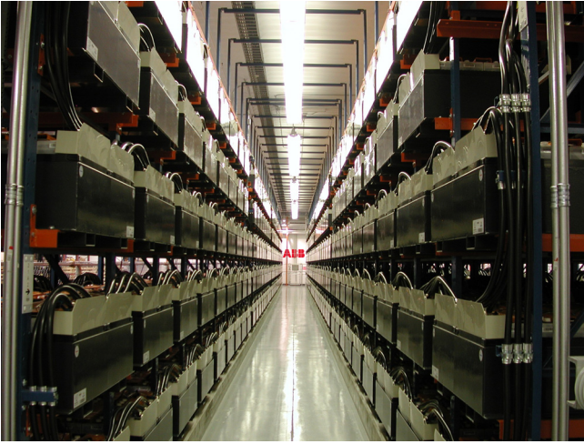
Figure 8.8 Inside view of large battery energy storage system (BESS), essentially a “substation size” UPS. It is housed in a small warehouse located at a utility substation. This facility provides 27 MW of power for about 15 minutes, enough to ride through a brief outage or fill in during a period of needed energy stabilization.
