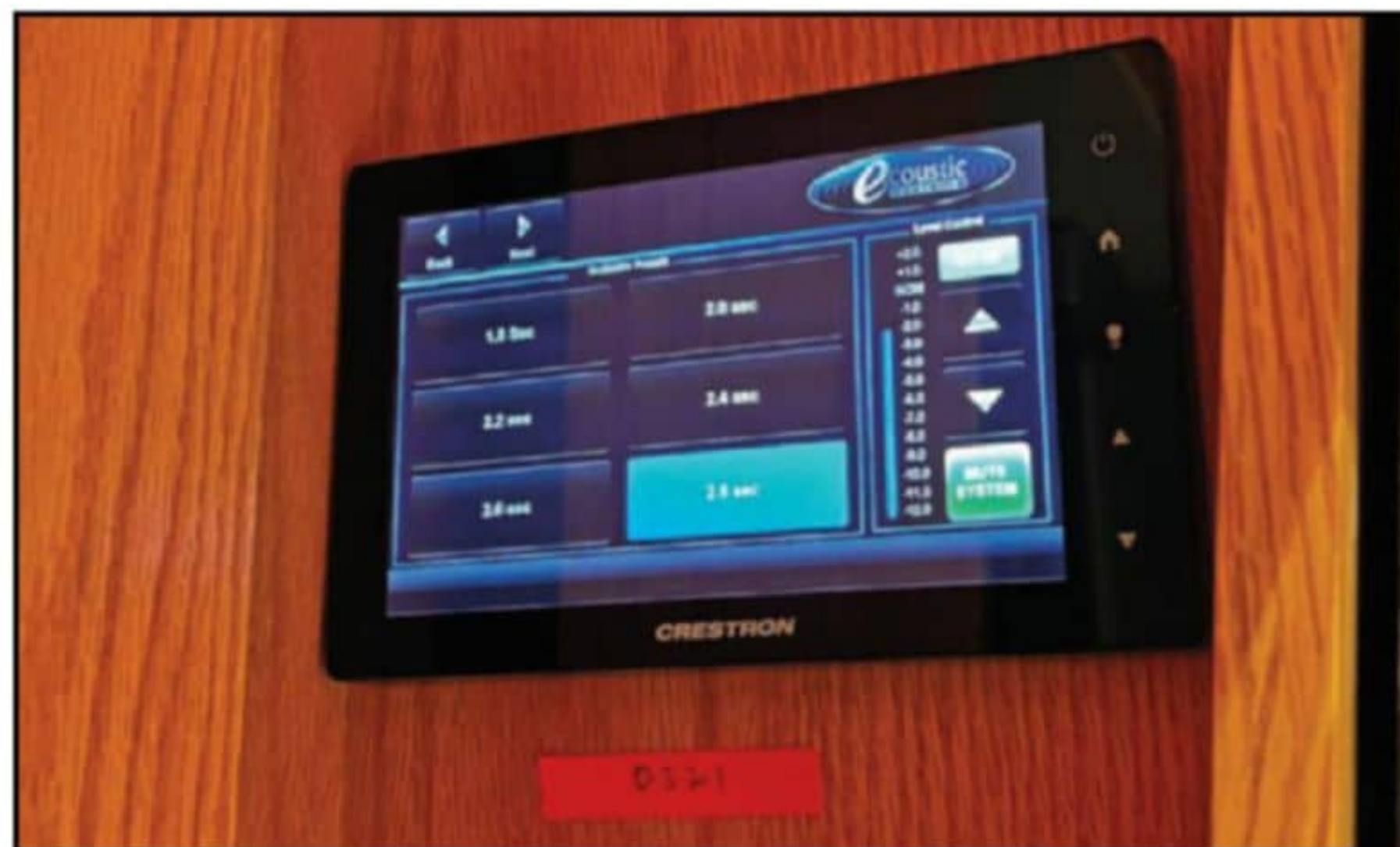
The E-Coustic Systems control panel placed on the doorway to Cary Hall allows full control by users of the active acoustics, according to the requirements and different usages of the room.
