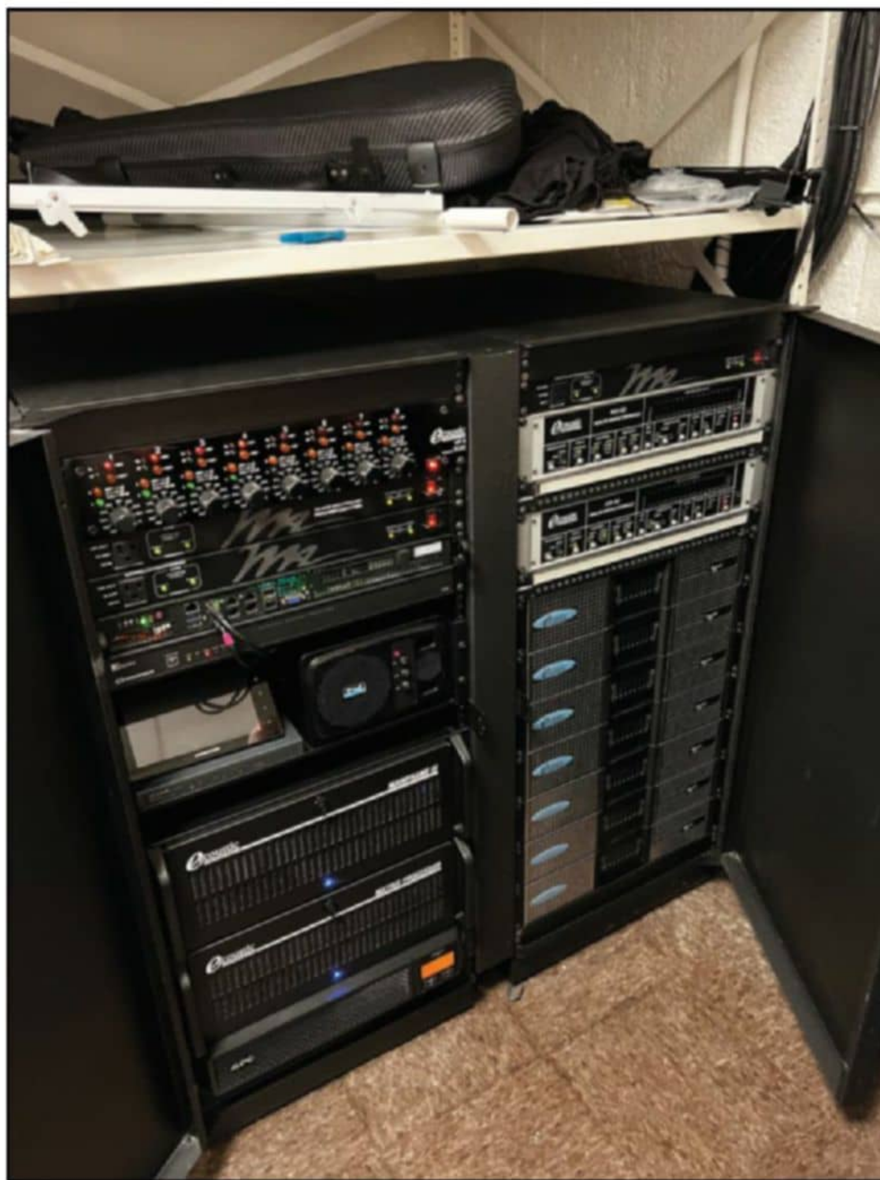
The complete E-Coustic Systems for the room active acoustics and all the auxiliary signal management is placed in these two half racks. The left side contains the E-Coustic Systems MP-8 Microphone Preamplifier, power conditioner, network router, Crestron control system, and the two main E-Coustic Mainframe III (that run all the advanced acoustics algorithms), and 512-channel Matrix Processor units. The right side is where the AO-32 Analog Output Interfaces provide the signal conversion from the digital processors back to analog balanced circuits, followed by the eight-channel power amplifiers that feed all the 56 speaker channels in the room.
