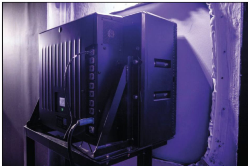
Figure 2: The X1 Matrix Array is shown in situ at Illuminarium Atlanta, placed behind a specially designed MDI panel.
