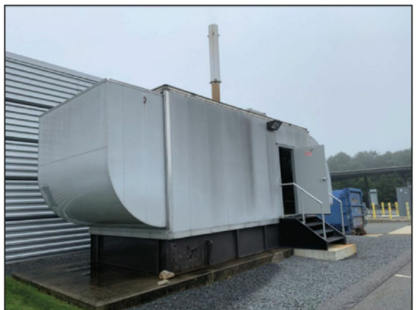
Photo 4: This diesel generator is the primary exterior noise source.
