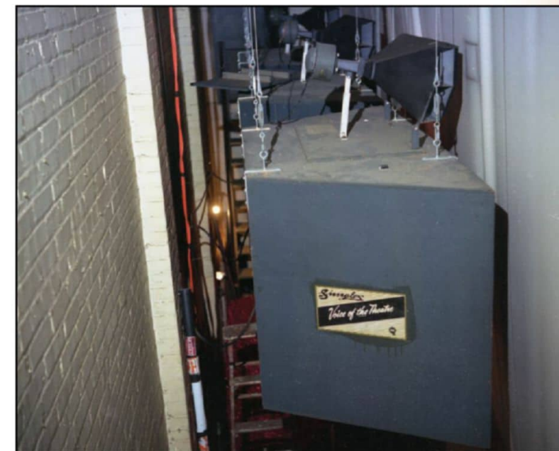
Other companies made cabinets based on Altec plans and filled them with Altec hardware. These A-5 cabinets were built by Simplex for very small Cinemascope installations.
