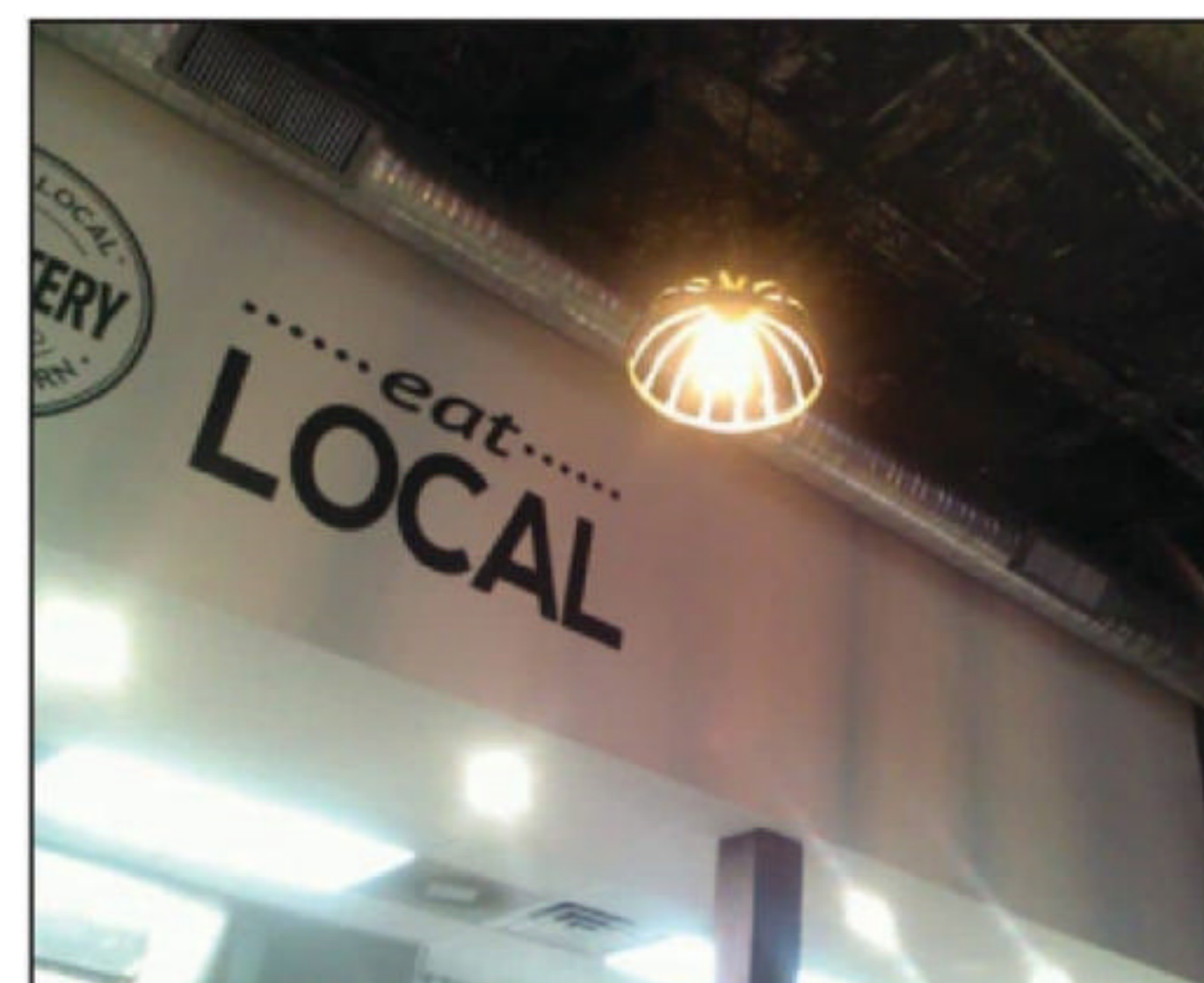
Photo 2: Air supply diffusers mounted directly to a duct are noisy.
