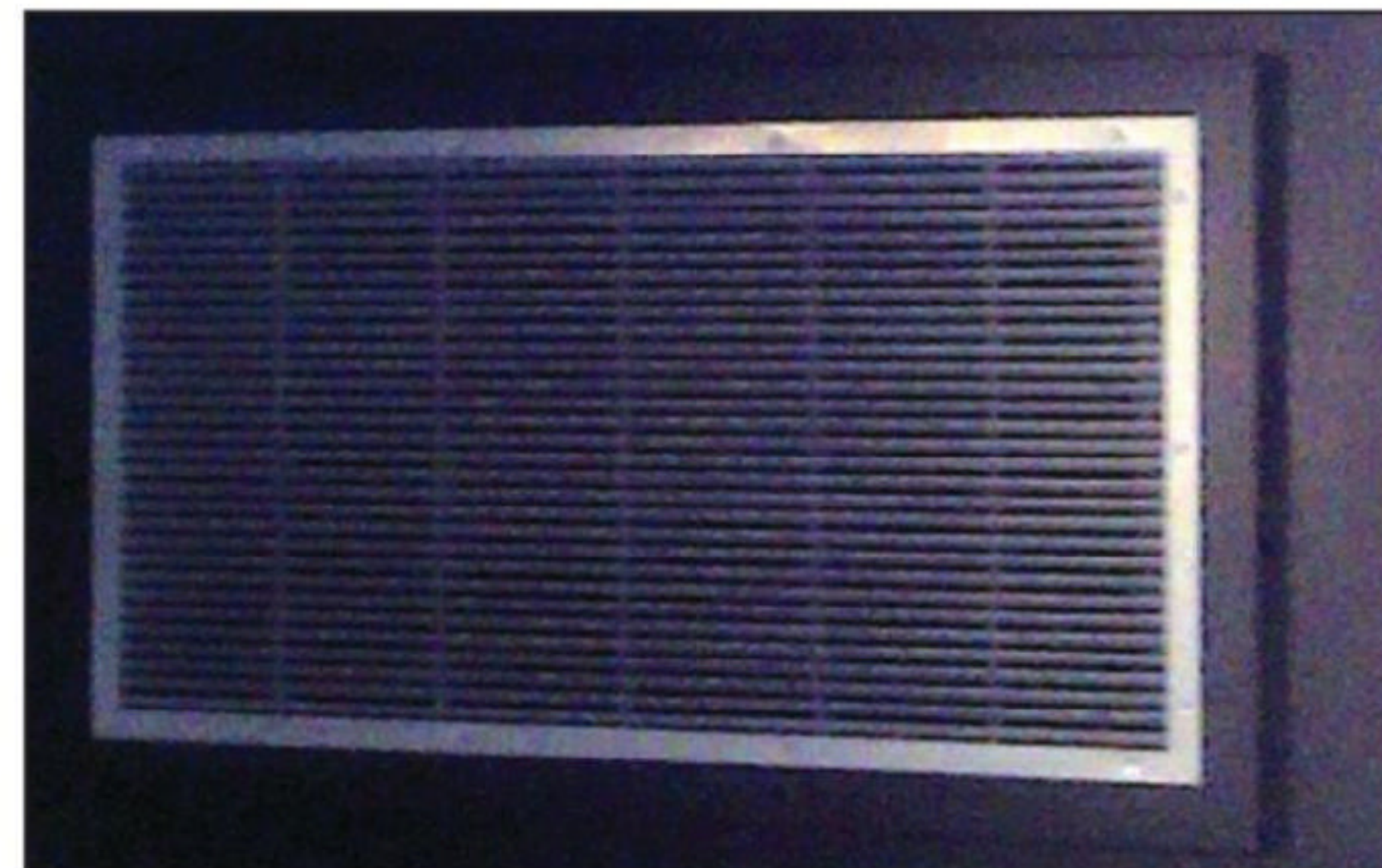
Photo 4: Return vents feeding directly to the AHU are noisy.
