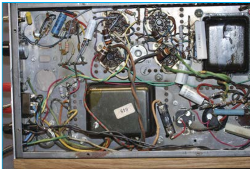
Photo 3: Much of the wiring had to be revamped.
