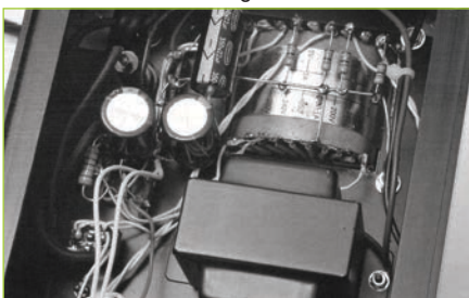
Photo 5: The power supply connections are shown.
