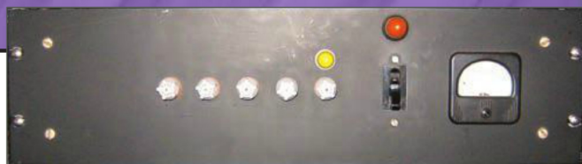
Photo 5: The power distribution
