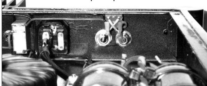
PHOTO 7: Closeup of the phase inverter switch S3.
