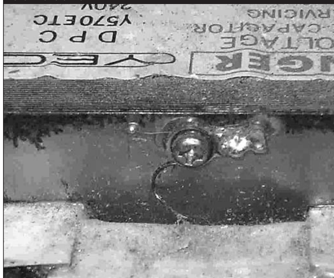
PHOTO 3: Close-up of the secondary earth contact on a microwave oven transformer.
