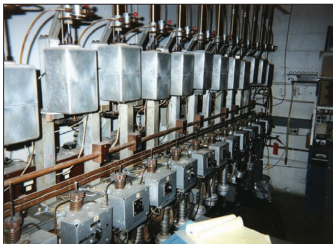
PHOTO 5: 12 station exhaust system. Used for 3D21WB and 7403 types.
