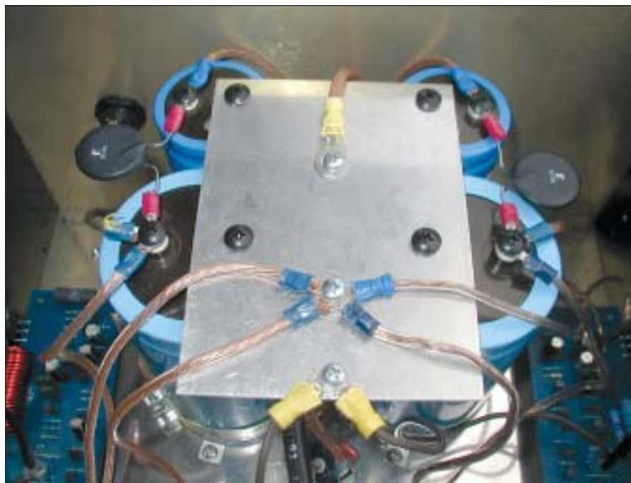
PHOTO 4: Grounding scheme of unit.
