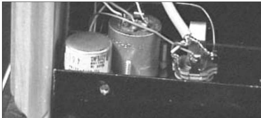
PHOTO 4: Closeup of input wiring.
