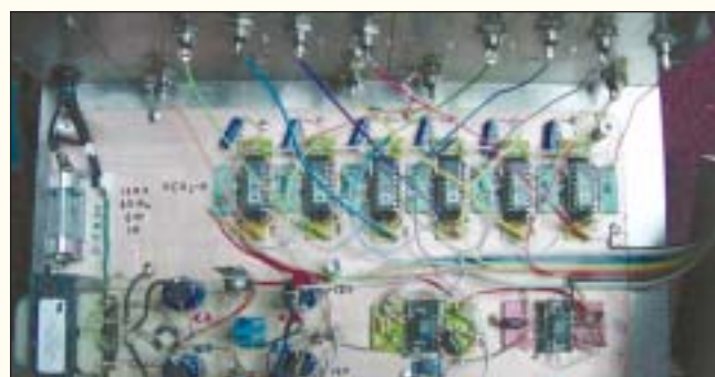
PHOTO 4: Inside the control.
